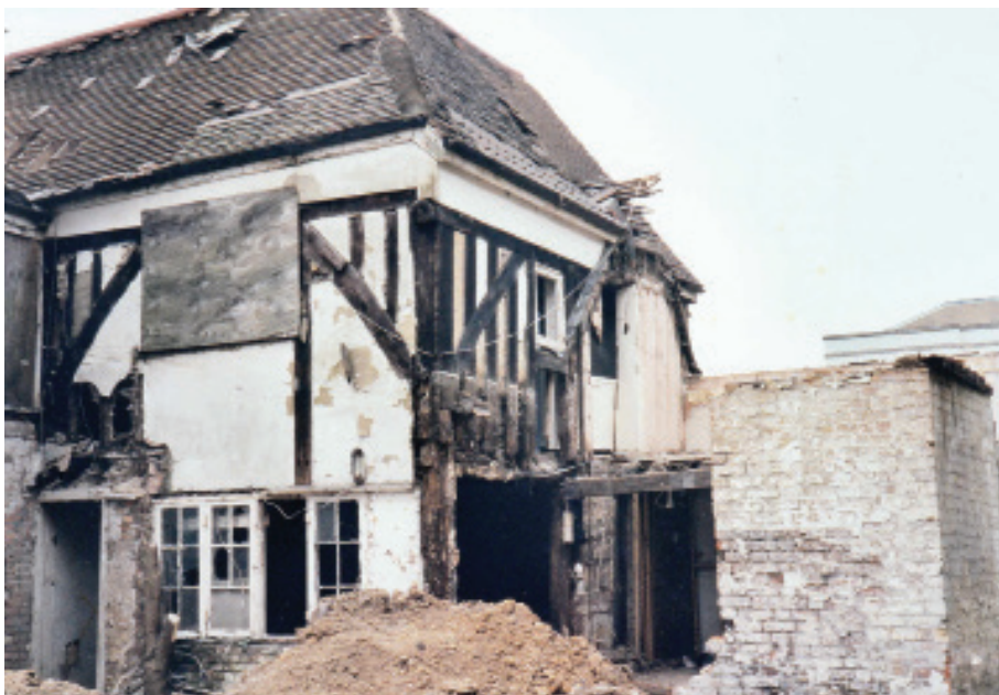
South-eastern corner of Phase-3 kitchen range with remains of later added range on right.
